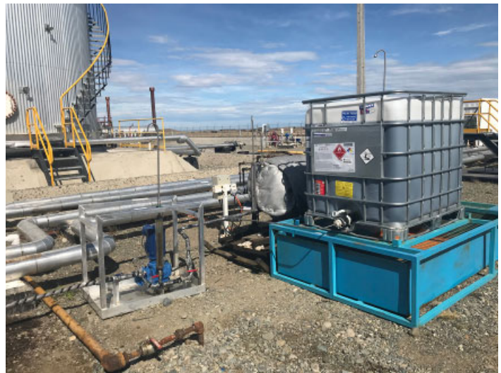
Chemical injection skid
