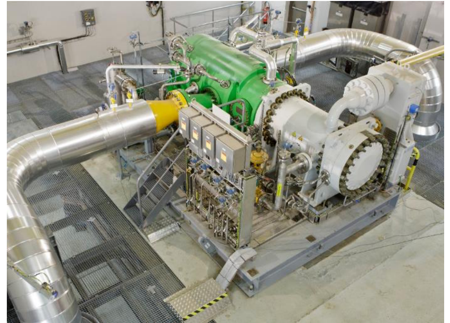
GRT Gaz Etrez site, France (© Philippe Dureuil)
