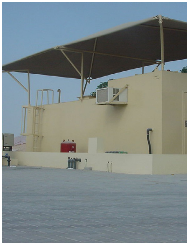
Water recycling systems like this one are examples of ways we are conserving water at our facilities
