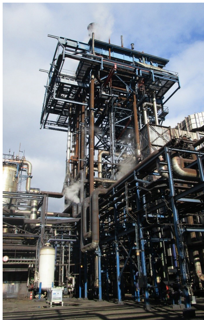
Figure 1 - Yara Tertre Steam Methane Reformer
